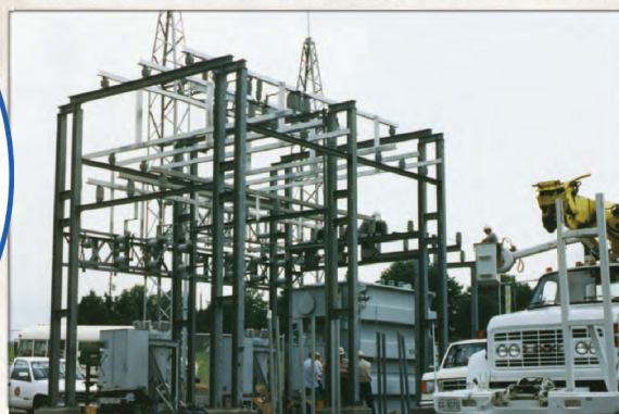
LEFT: Parkway Substation
